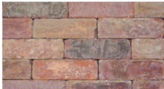
No Mortar Joint (Dry-Stacked)
